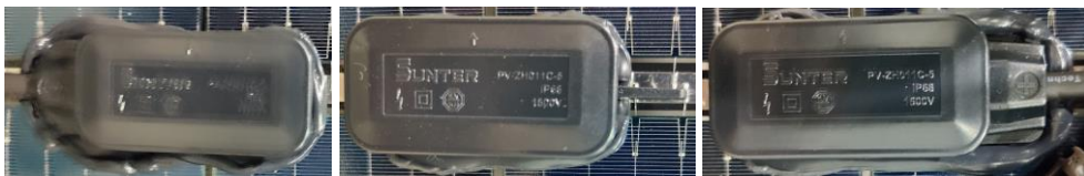
Fig. 05: view of junction box
