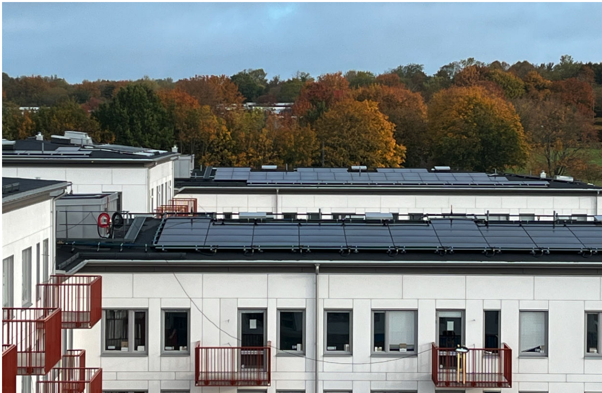
Swedish Magnolia apartment buildings development in Lund where the PV-T + Heat Pump energy system designed by Kraftringen lowers the carbon footprint achieved with district heating alone. This DualSun solar installation combines 168 PV-T and 150 PV panels.
